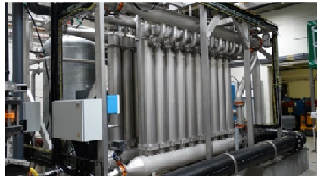
Ceramic Microfiltration In 'waste water area'
