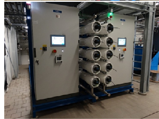
RO installation in 'Drinking water area'. At borders feed and permeate tanks. IBC tanks for chemical cleaning.
